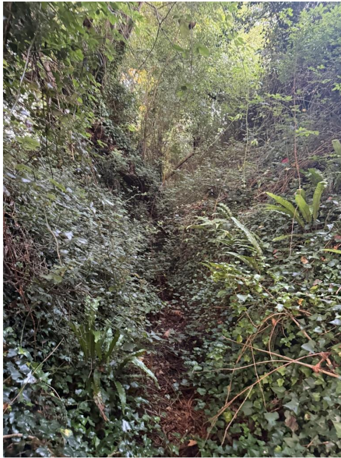
Plate 2. Vegetated drainage ditch
